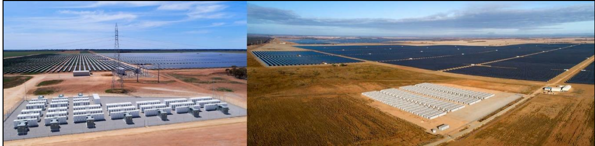
Figure 10.2.7 – General examples of BESS alongside solar farm
