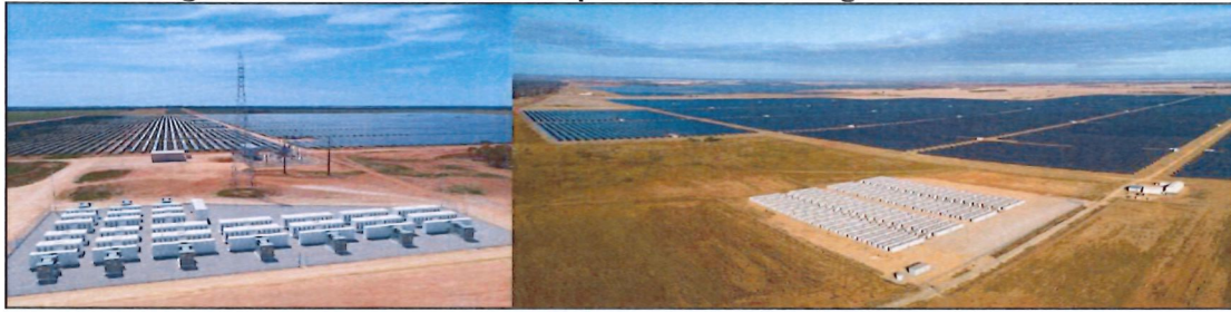
Figure 12.2.8 – General examples of BESS alongside solar farm
